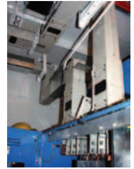
把电站直接连到母排 direct connection from substation to busbar
