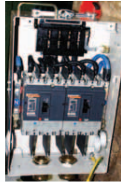
带有两个断路器的终端头 Tap-off with two circuit breakers
